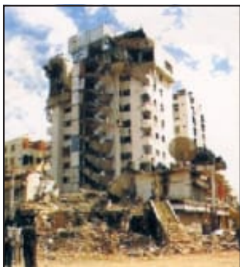
Fig. 3.3a: Destruction caused by an Earthquake in Gujarat
